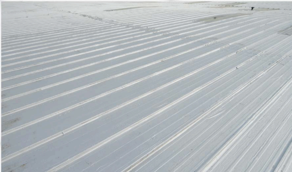
Metal covering after the final treatment - a coat of VERNICE ALLUMINIO has been applied 20 days after the second coat of EASYGUM (apply by spray; total consumption: 200 g/m 2 )
